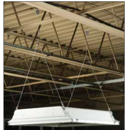
High Bay Lighting
