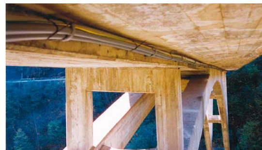
Bundled pipes and cables with one CLIC clamp at the underside of the Ponte Val Calanca bridge in Switzerland.
